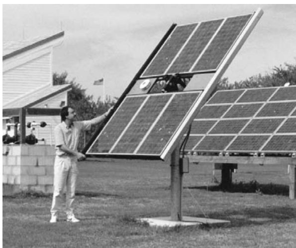
Figure 6.21 A pole-mounted array on a passive tracker at the Florida Solar Energy Center.
