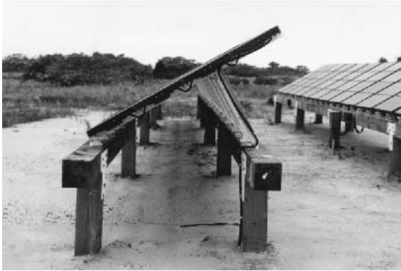
Figure 6.19 A ground-mounted array field using rack supports.
