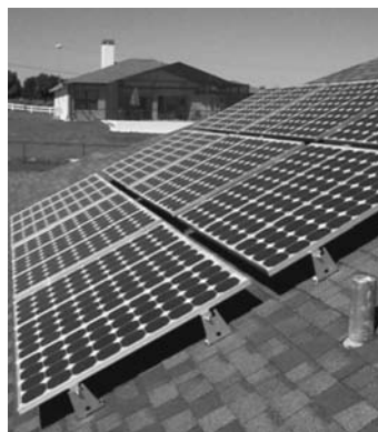
Figure 6.14 Standoff-mounted array installed using slotted roof brackets. These point connections and the standoff height promote good air movement between the roof and the back surface of the modules [FSEC photo].
