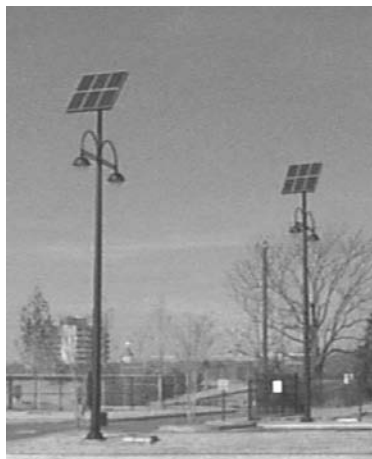
Figure 6.20 Pole-mounted arrays are often used for PV lighting systems.
