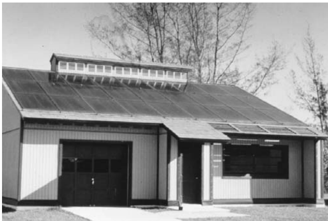
Figure 6.17 For this experimental prototype, photovoltaic modules replaced conventional roofing materials.
