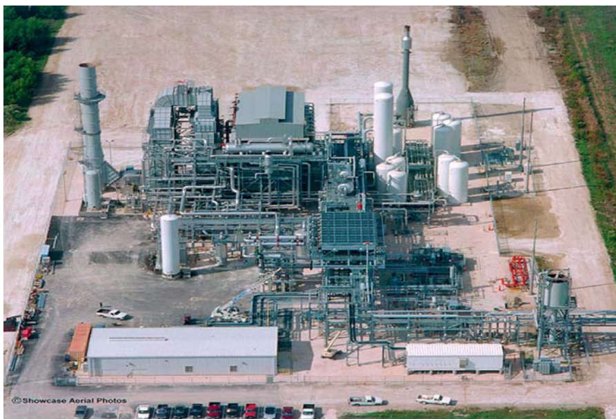
Figure 10.2. Aerial photo of Air Products and Chemicals, Inc.; an 80MMSCFD H 2 plant in Pasadena, TX (SMR H 2 facility and 10-bed H 2 PSA).
