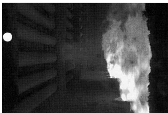
Figure 15.23 Crude unit burners. (From Ref. 31. Courtesy of John Zink Co. LLC.)
