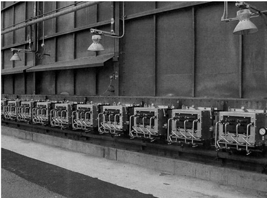
Figure 12.35 Ultra-lean premix burners installed in a process heater. (Courtesy of John Zink Co. LLC, Tulsa, OK.)
