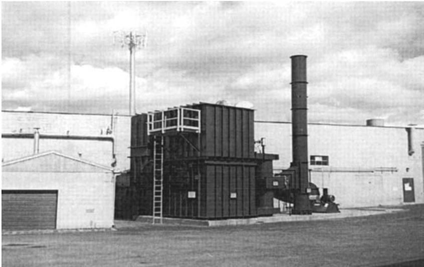
Figure 7.27 Regenerative thermal oxidizer. (Courtesy of Alstom.)
