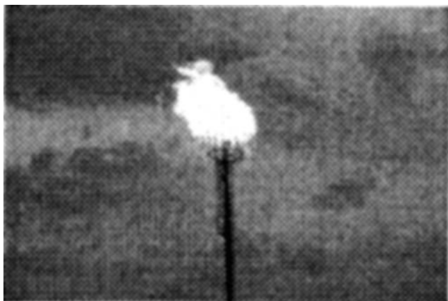
Figure 15.32 Typical elevated multipoint flare system. (From Ref. 63. Courtesy of John Zink Co. LLC.)
