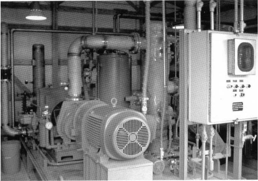
Figure 17-4. Gas Compression System
